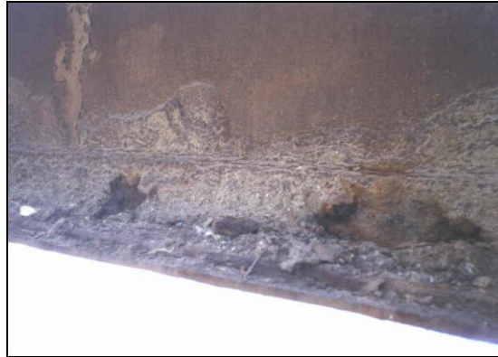
Figure 28. Photo. Heavy corrosion of bottom flange and web due to collection of poulitce.
