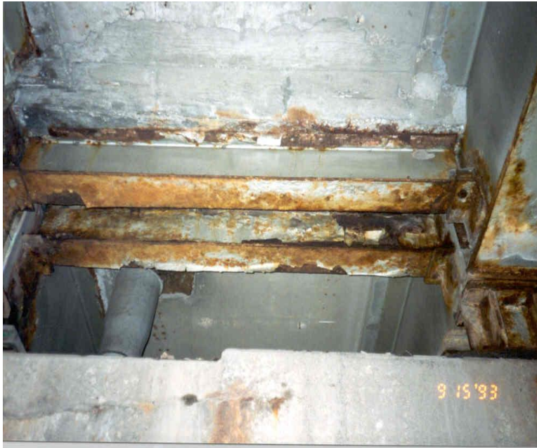
Figure 16. Photo. Steel directly beneath transverse expansion joints that have leaked corrosive runoff from the deck.
