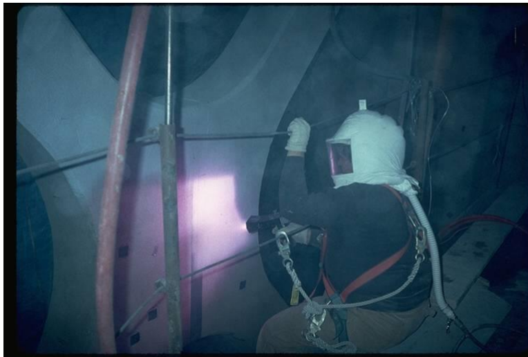
Figure 5. Photo. Metalizing of a bridge member in the field (photo courtesy of R. Kogler).
