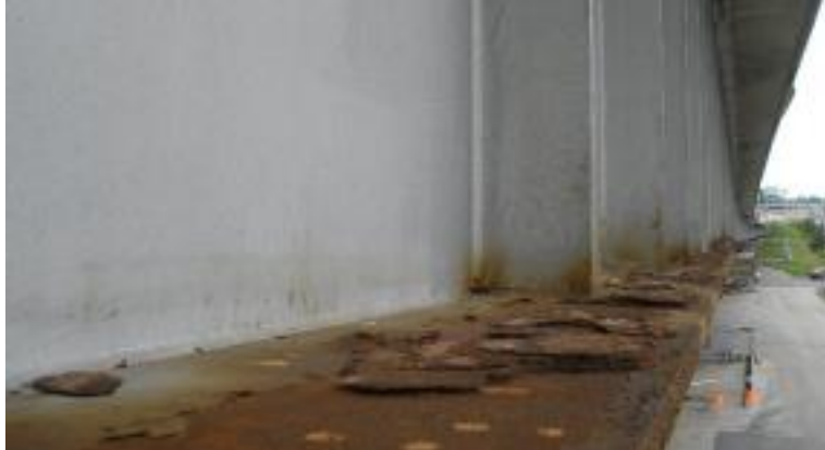
Figure 27. Photo. Corrosion localized to upper surface of lower flange, the rest of the bridge is fine.
