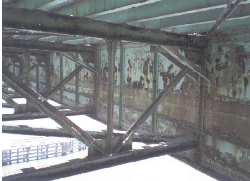
Figure 20. Photo. The area under an open grid deck acting as one large leaking joint.
