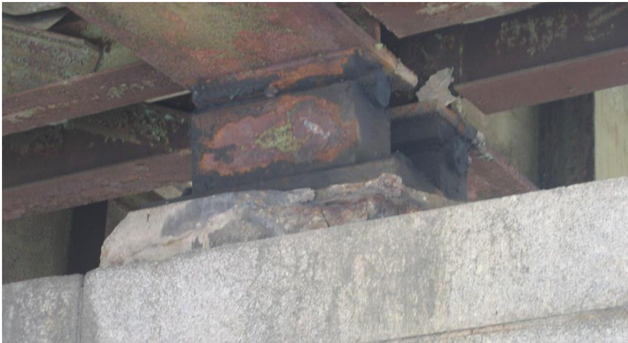
Figure 30. Photo. Corroded bearing.
