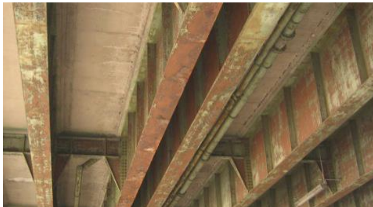
Figure 19. Photo. Closely spaced girders lead to difficult access for maintenance activities.
