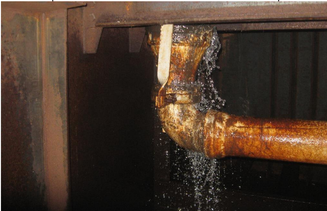
Figure 22. Photo. Clogged drain leaking water onto superstructure.
