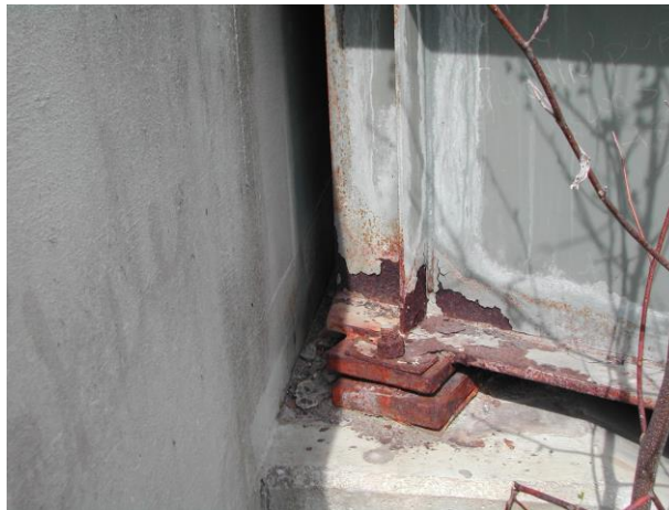
Figure 15. Photo. Deterioration of bearing area beneath a leaking joint with only single-coat inorganic zinc-rich paint.
