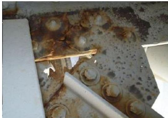
Figure 38. Photo. Corroded lateral gusset plate detail.
