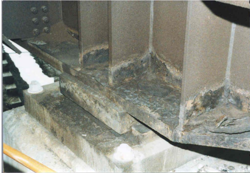
Figure 34. Photo. Girder end on a bearing below a leaking deck joint. Horizontal flange and vertical stiffeners create an excellent trap for debris and moisture.
