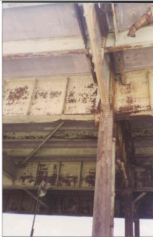
Figure 21. Photo. Missing portion of deck drain downspout.
